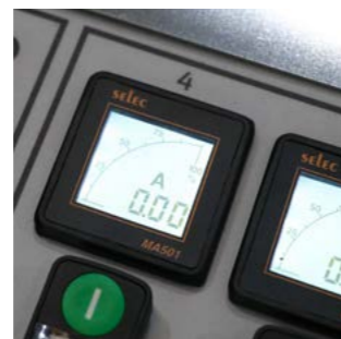
__ mobile control panel
